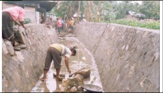
Improvement of main outlet drain of ward No. 8,9,12 and 13 and sluice gate provision
