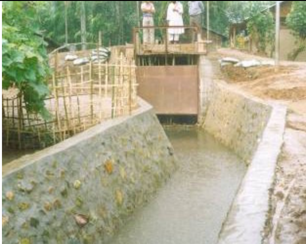
Construction of pucca drain with RCC culvert cum sluice gate near Deepchand Rajkhowa Road
